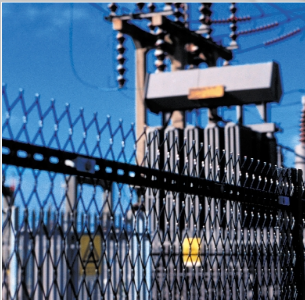
High security protection of sub stations
